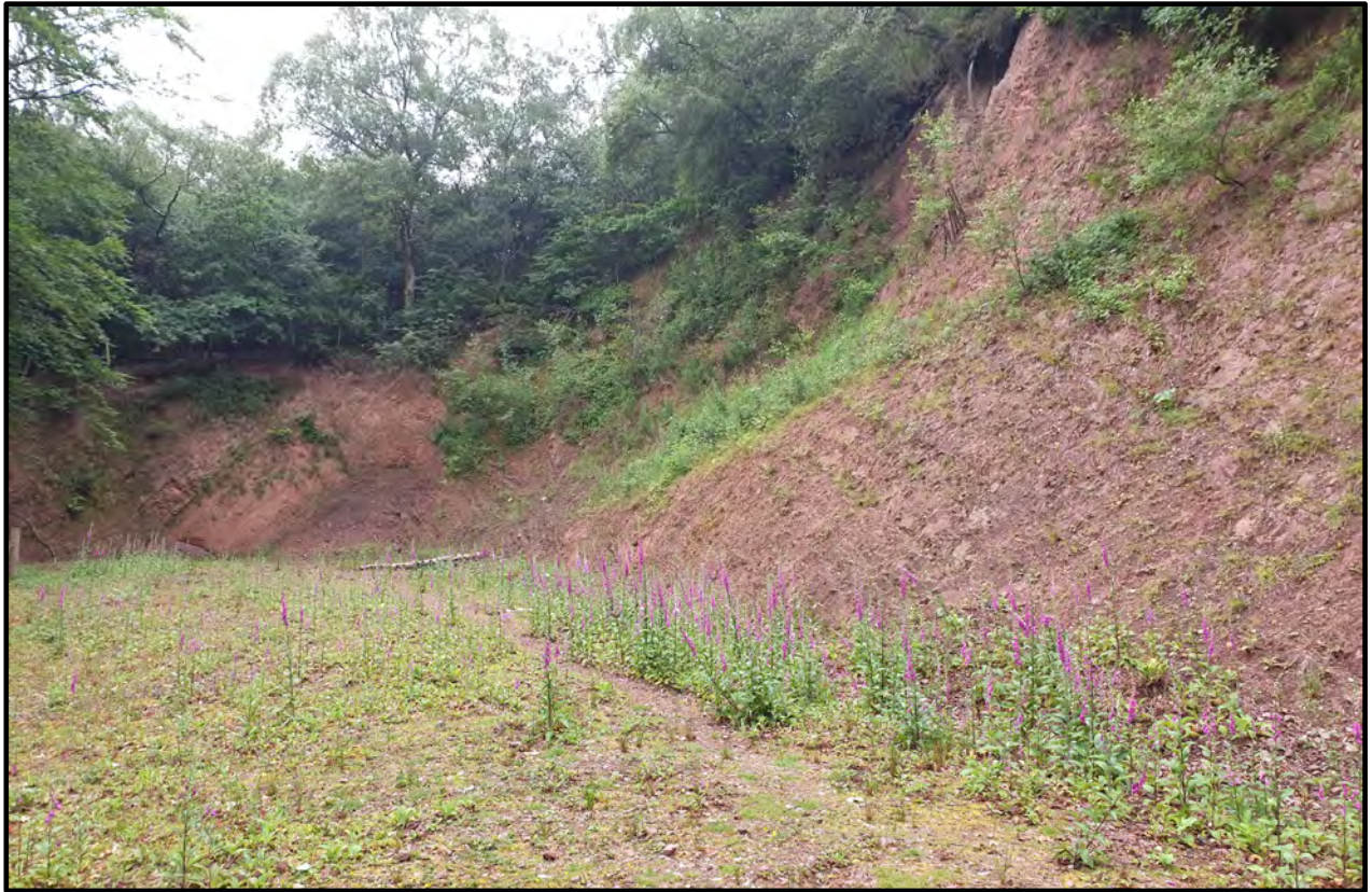
Photograph 13. SP001753 June 2020 Overhanging trees and encroaching vegetation is obscuring the structures unique to this locality. [June 2020 Malcolm Coghill]
