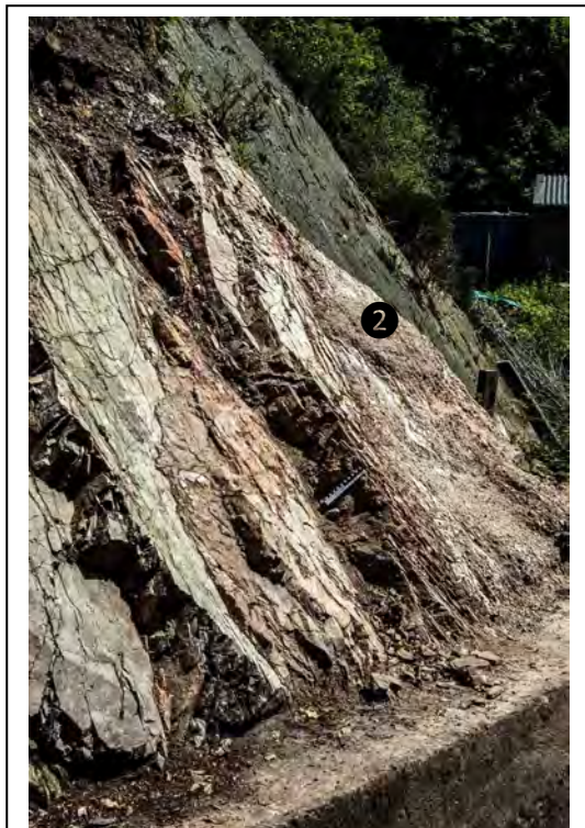
Figure 2 – 2019: The fissure infill above the NW wall of the ammunition store.
